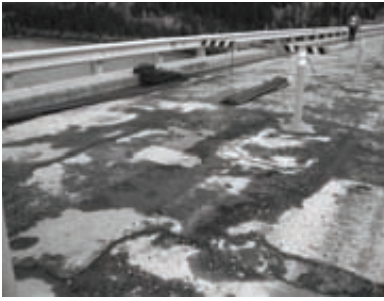
Many bridges in the Yukon require major rehabilitation to bring them up to minimum standards.
