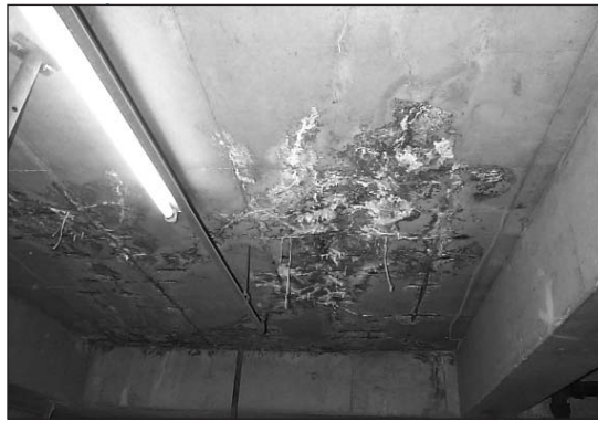
Deterioration on underside of parking garage floor prior to rehabilitation
