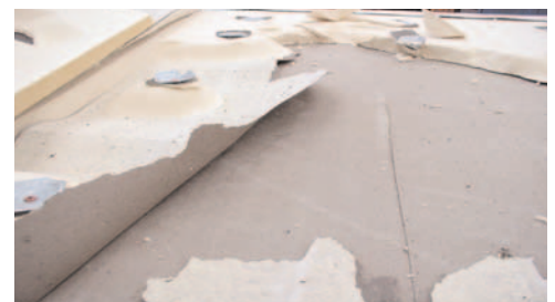
Fully bonded system after wind testing showing failure modes in the insulation and adhesive
