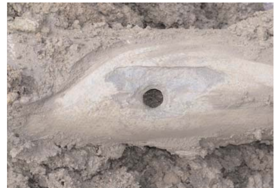
Service connection pull out
