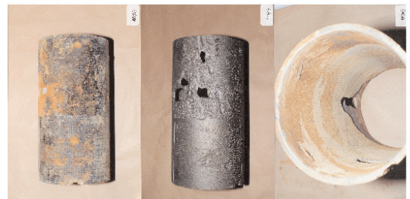
Corroded ductile iron mains
