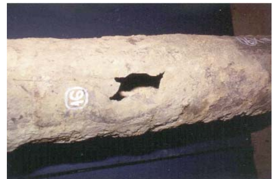
Failed cast iron distribution main
