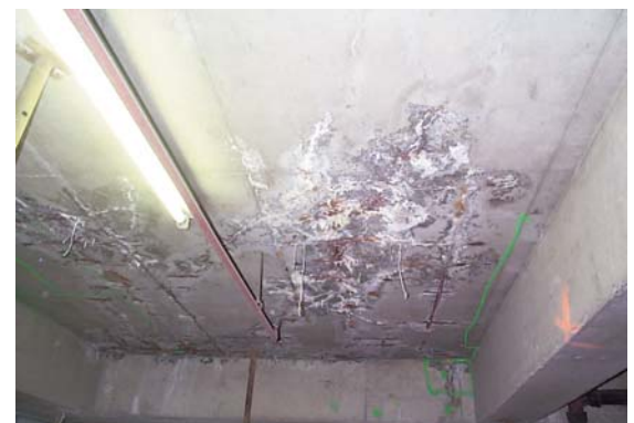
Underside of concrete slabs at the Laurier-Taché parking garage before rehabilitation
