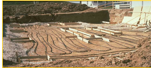
Ground Source Heat Pumps
