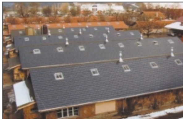
Atlantis Solar Systems SUNSLATES™, used for residential roofing systems in Berne, Switzerland.
