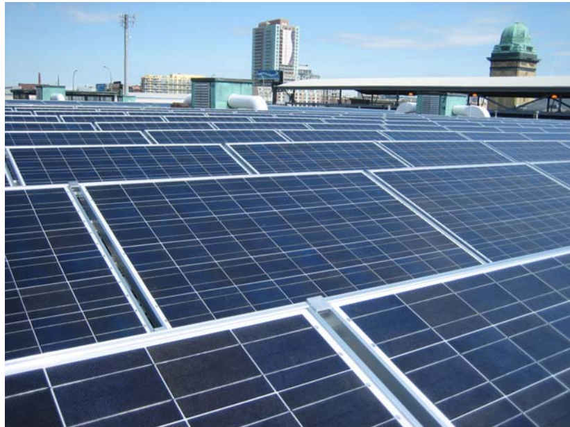
Fig. 1: 1100 kW PV roof-mounted installation at exhibition Place, Toronto, Ontario, Canada. (Photo credit Exhibition Place)
