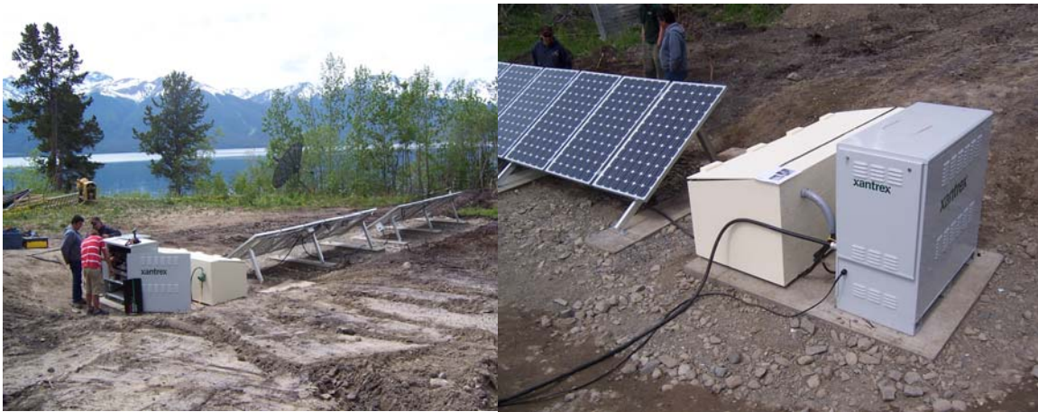
Fig: 3 The Xantrex Hybrid Power System reduces First Nations generator fuel consumption and increases reliability at a remote site (Photo credit Xantrex)
