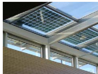
Fig. 2: Skylight systems at the Fred Kaiser Building, UBC, British Columbia, featuring a grid-tie 7 kW BIPV. (Photo credit Carmanah)
