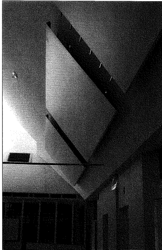
Radiator panels, shown mounted on the cathedral ceiling, provide both heating and cooling.
