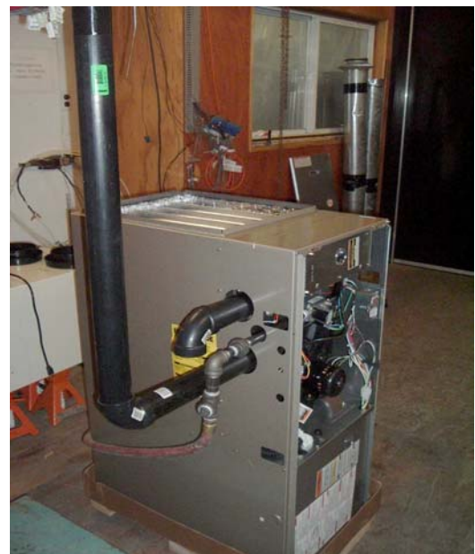
Figure 11 - High Efficiency Furnace Vent Configuration Showing Combustion Air Intake Sample No. 04-06-M278-6
