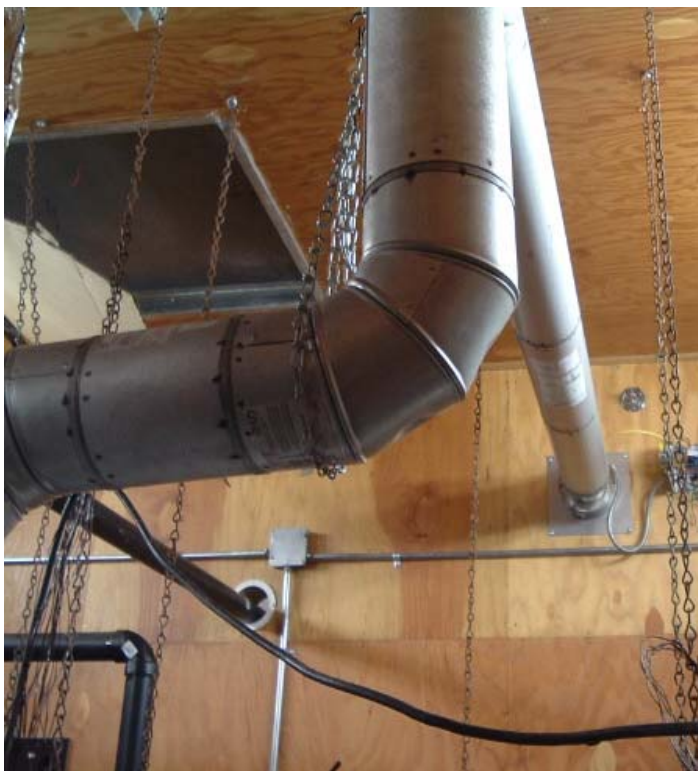
Figure 3 – Mid-Efficiency Furnace 'Type B' Vent Configuration Sample No. 04-06-M0278-2
