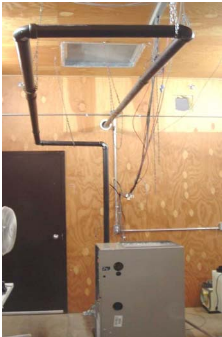
Figure 10 - High Efficiency Furnace Vent Configuration Sample No. 04-06-M278-6
