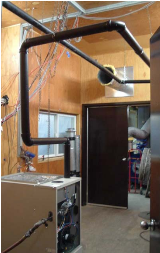
Figure 8 – High Efficiency Furnace Vent Configuration Sample No. 04-06-M278-5
