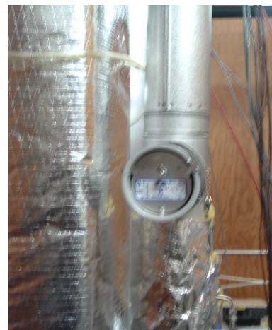
Figure 4 – Barometric Damper Location Sample No. 04-06-M0278-2
