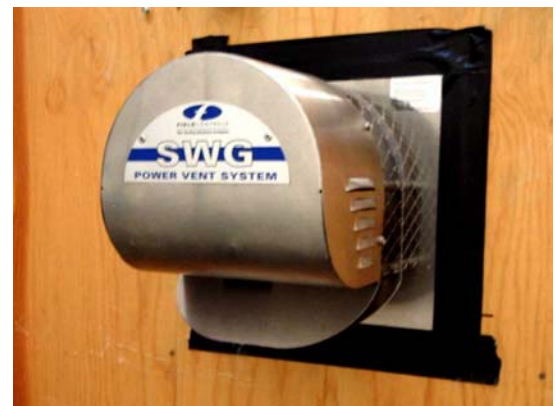
Figure 5 – Power Venter Exhaust Terminal Sample No. 04-06-M0278-2
