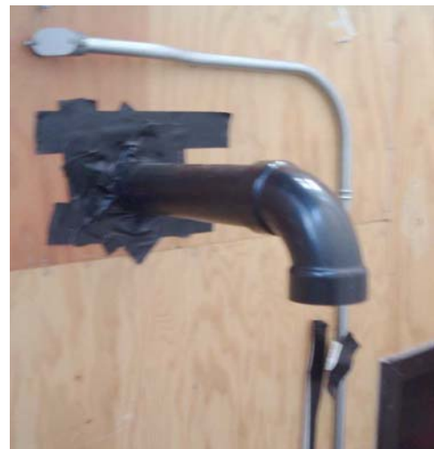
Figure 7 – Exhaust Terminal Sample No. 04-06-M0278-4
