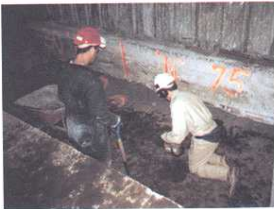
Monitoring for residual contamination after removal of contaminated soil from beneath a building at the Anvil Way site in Surrey.
