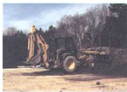
Contaminated soil is shaped at the working area of the Temporary Storage Site in Port Hope.
