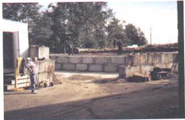
Completing the expansion of the storage bunker at the Anvil Way site in Surrey.
