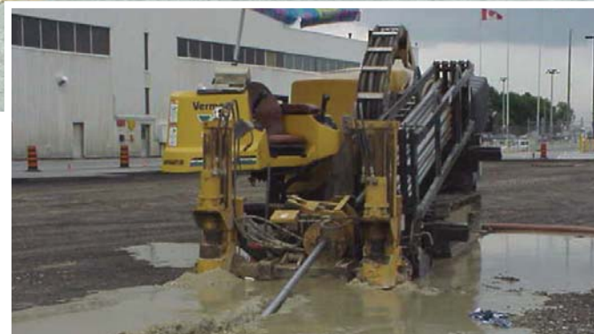
PWGSC's use of a directional boring machine to install lighting onto airport pavement was an innovative way to save time and money.
