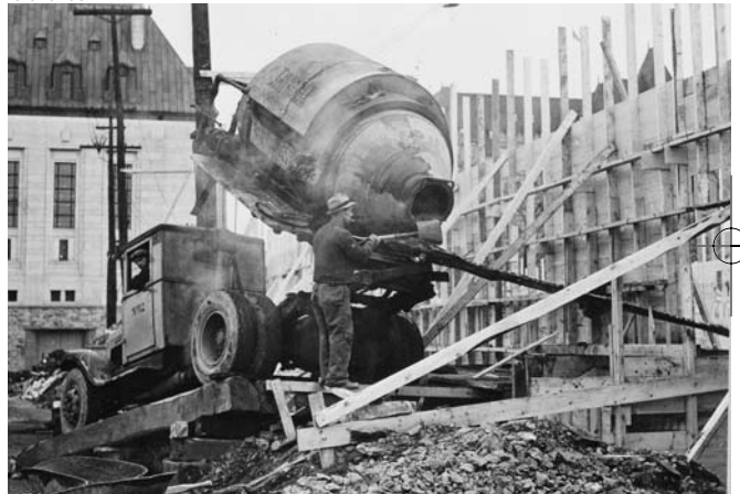
Construction work begins on Temporary Building Number four – being built to accommodate expanding wartime government departments.
