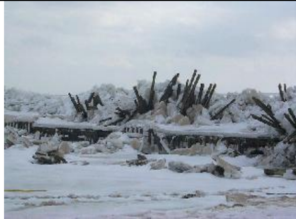
Photo 3. Ice pile-up at Cap-des-Caissie wharf.
