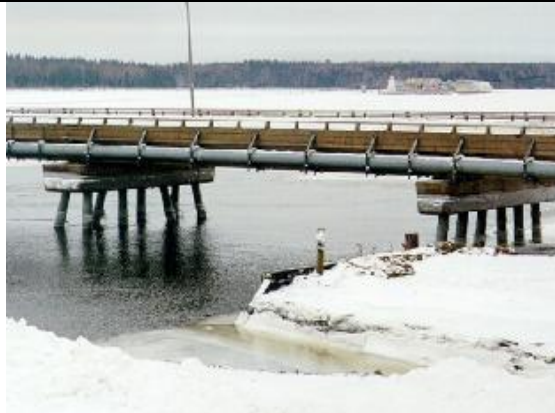
Photo 13. Wetting line at Bouctouche.
