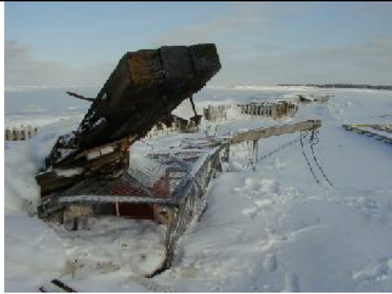
Photo 8. Ice damage at Robichaud.
