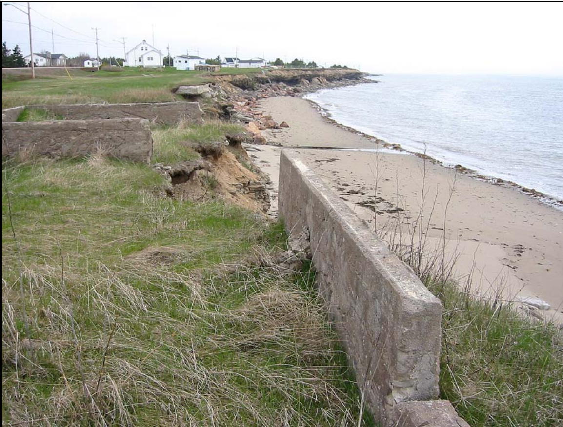
Figure 2. Foundation of an abandoned fish plant south of Cap Lumière, partially destroyed by erosion of low sandstone cliff (D.L. Forbes/GSC, May 2005).
