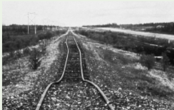
Changes in ground surface due to melting permafrost can affect the stability of structures.
