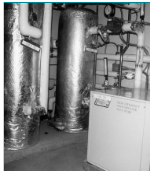
A single heat pump with buffer and heating tanks.
