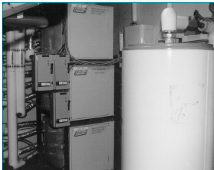
Multiple heat pumps with domestic hot water preheat tank.
