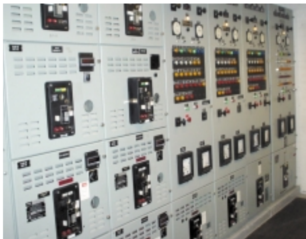
Control centre in the Health Region
