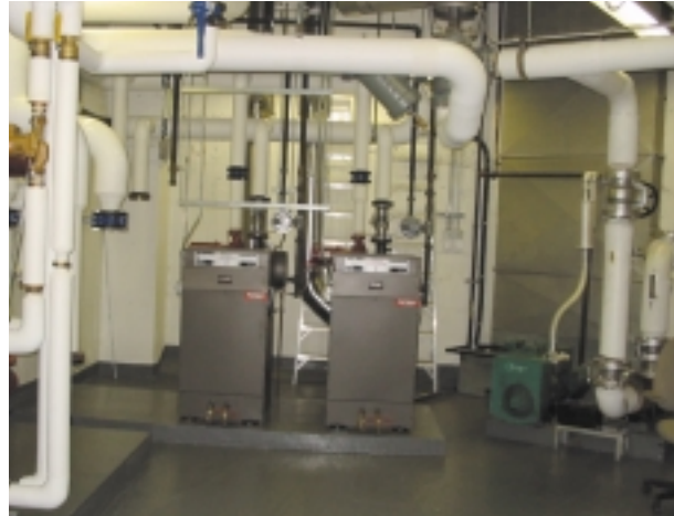
New furnace system at Hendry House
