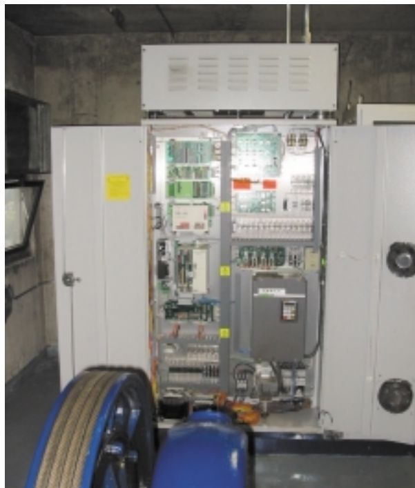
New elevator system
