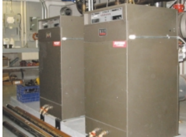
New furnace system at Central Plaza
