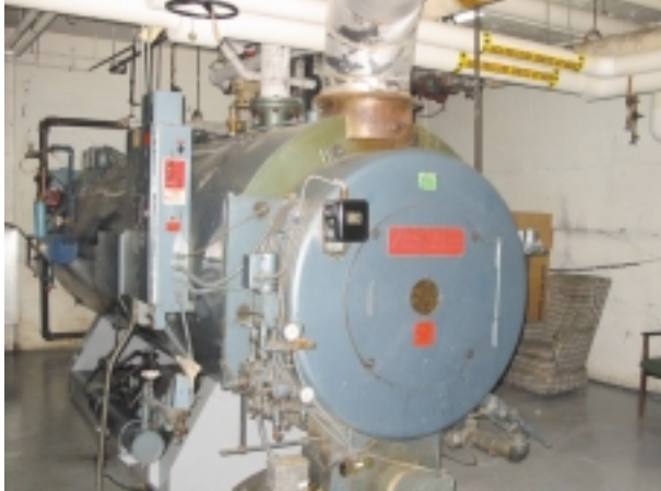
Old furnace system at Central Plaza
