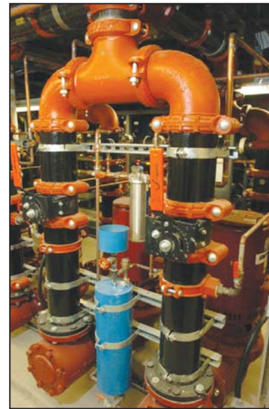
Figure 16: Secondary loop pumping system for recovery of heat rejected by the refrigeration systems in a supermarket.
