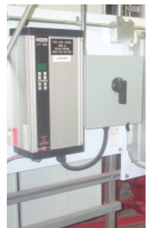
Figure 1 – Typical Variable Frequency Drive Control Panel
