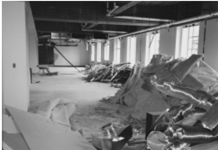
PWGSC encourages practices which reduce the amount of demolition materials sent to landfills.
