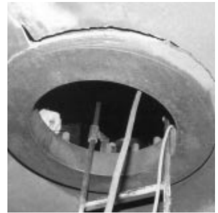
Pre-cracks on the surface of the manway plate
