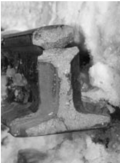
The rail fractured at a thermite weld
