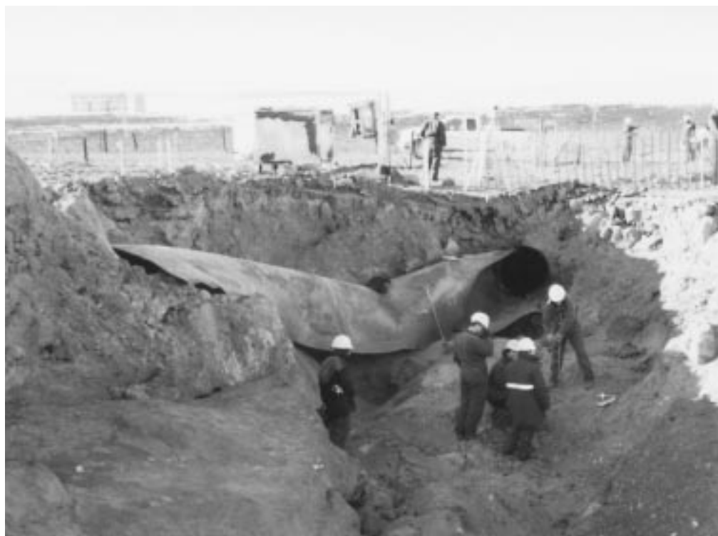
Ruptured pipe on Line 100-3 near Cabri, Saskatchewan.
