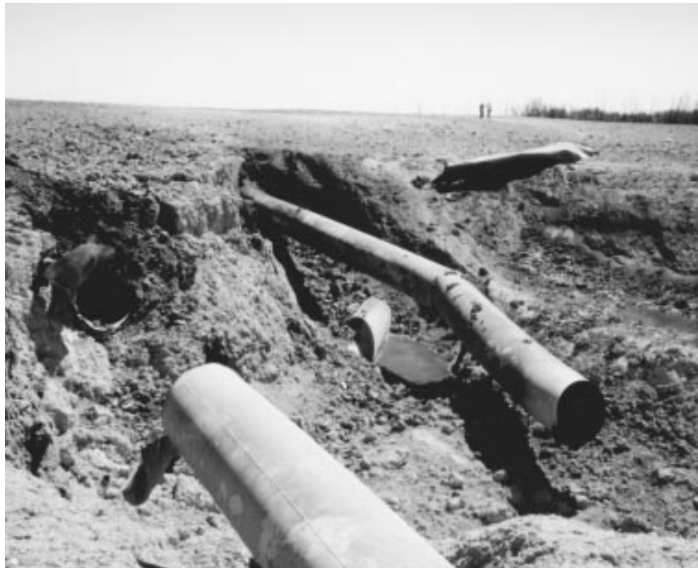
Ruptured Lines 100-3 and 100-4.
