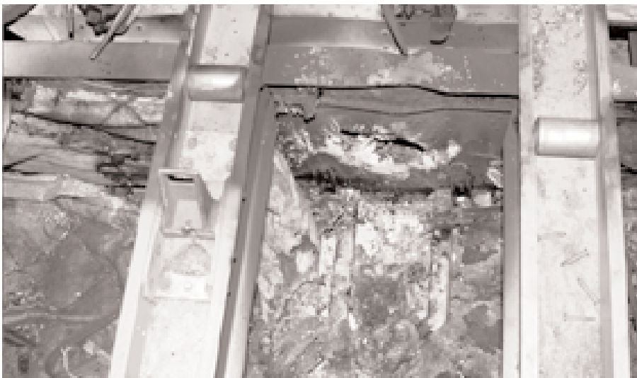
Fire damage caused by a faulty water-line ribbon heater. Note the heat-induced distortion to the beam structure.
