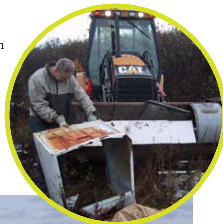
Heavy equipment, provided by Gulf Operators and the City of Saint John, helped remove tonnes of construction and demolition waste.
