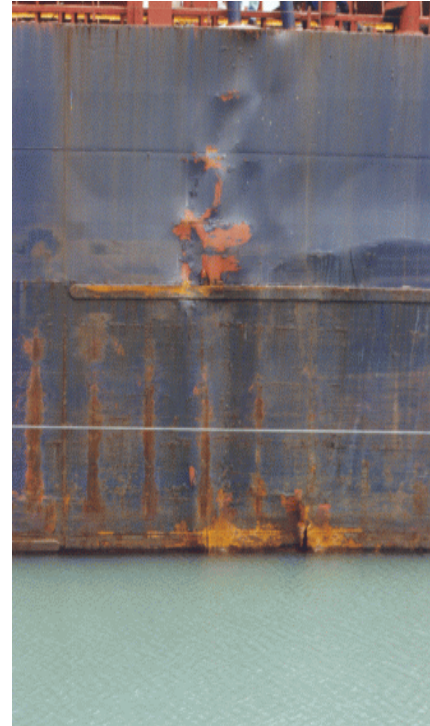
Photograph 2. Buckling and fractures on starboard side
