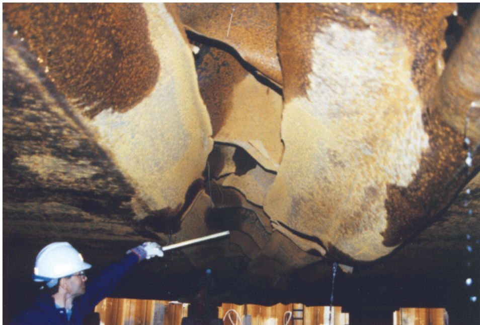
Photograph 4. Fracture damage to bottom plating in way of the transverse bulkhead between frames 117 and 119
