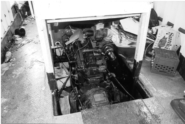
Photo 4 Opening in main deck with no steel coaming in way of portable plywood panels of engine casing.
