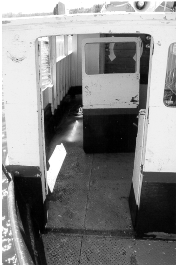
Photo 11 Opening in bridge front with stove-in door forced inside superstructure and unpainted, corroded foot print on main deck of missing door sill.
