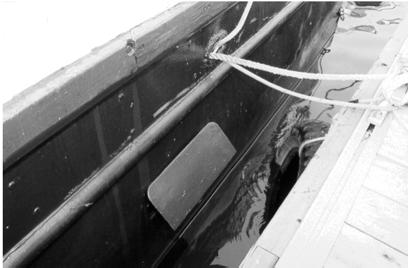
Photo 6 Main deck freeing port in hinged open position.
