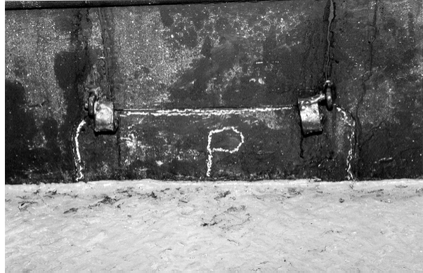
Photo 7 Main deck freeing port welded shut. Starboard side is similar.
