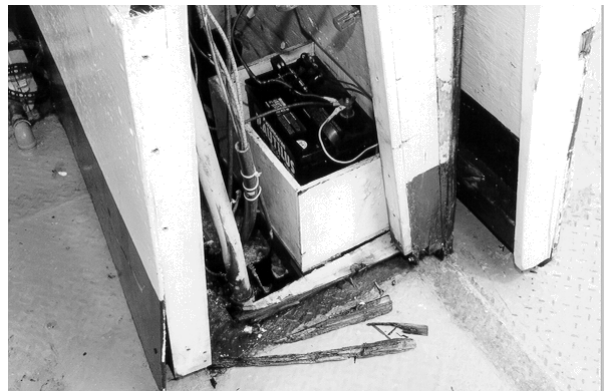
Photo 9 Disintegration due to dry rot of door frame and console base, and corrosion in way of irregularly shaped hole in main deck.
