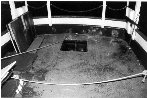
Photo 2 Aft end of main deck showing intact steel bulwark and hatch opening in main deck with no sealing gasket or means of securing flush wooden cover.
