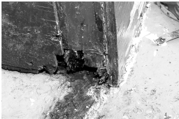
Photo 10 Disintegration due to dry rot of inboard base of bridge front door frame (outboard base similar).
