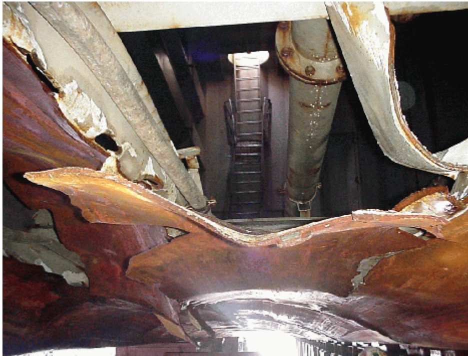
Photograph 2. Bottom damage to the MV Mokami
