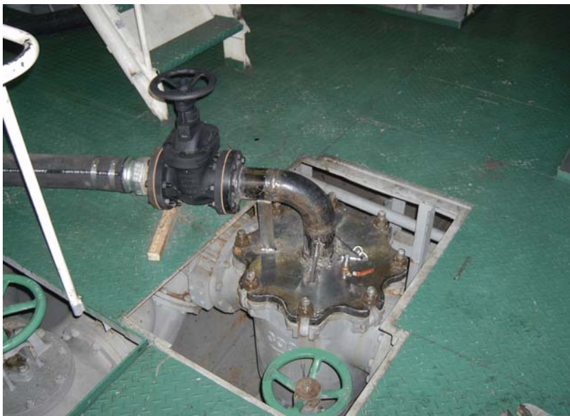
Photo 4. Temporary pipe connected to sea strainer returning main engine cooling water directly to sea chest.
