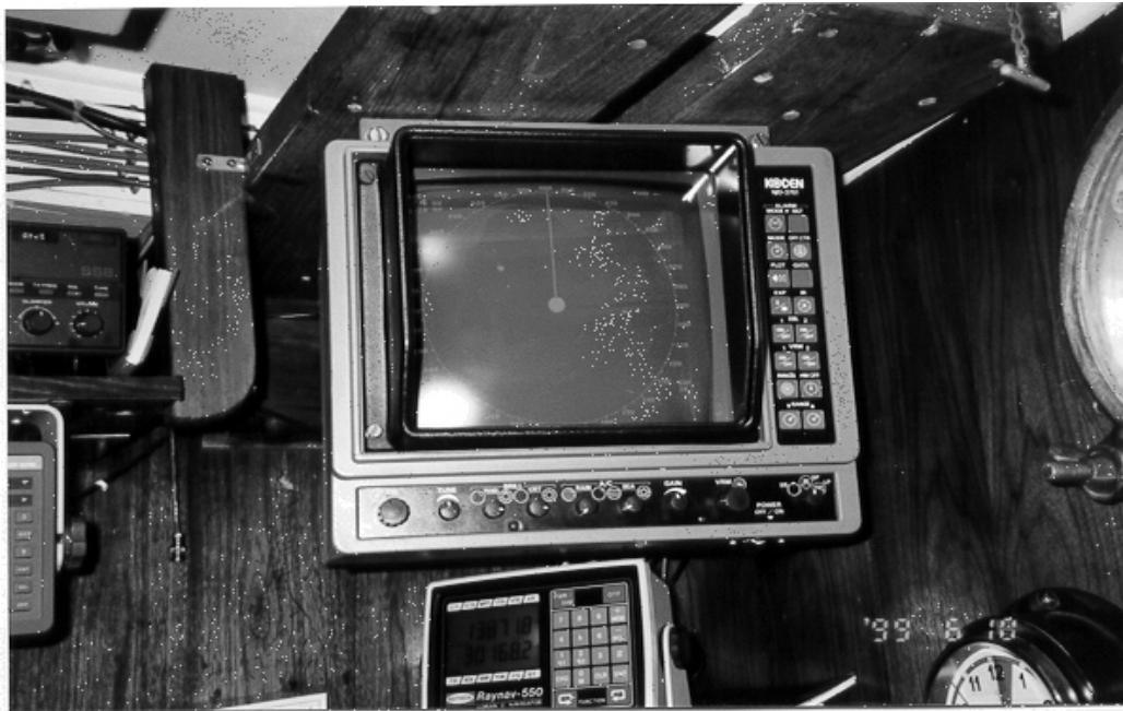
Radar display in the chart room—not visible from the conning position
