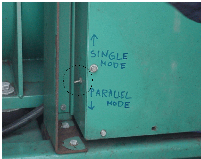
Figure 1 - Toggle switch mounted on temporary genset control panel
