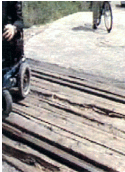
Figure 2 -The crossing planking was in very poor condition.
