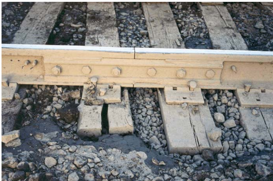
Photo 3. Close-up of joint north of Highway 12 crossing
