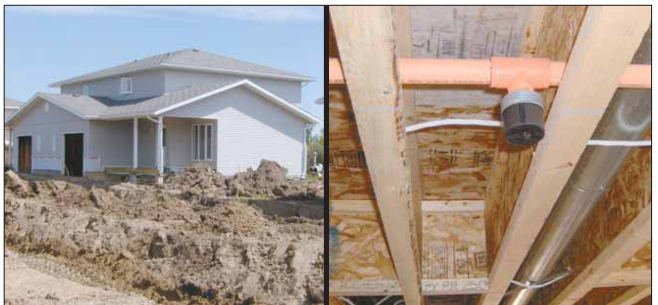
DND Housing Units under construction at CFB Wainwright, Alberta incorporating the installation of residential sprinklers.
