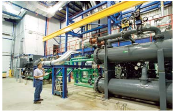
Compressors CMP1 and CMP2
