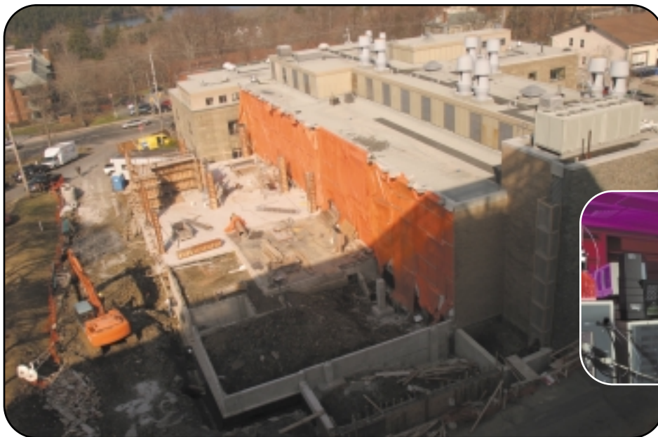
Construction of the new Industry Partnership Facility at NRC-IMB in Halifax began in early 2003 and is slated for completion by the end of the year.
