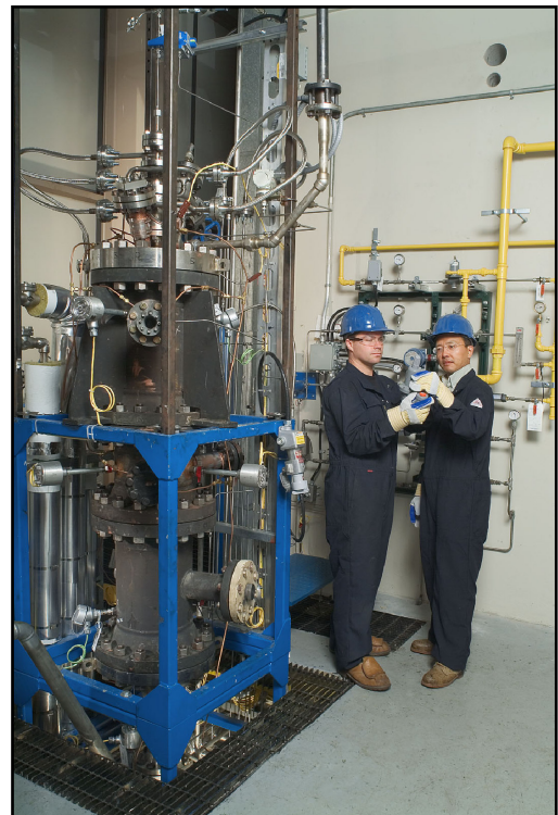
CEPG's PRESSURIZED GASIFIER
