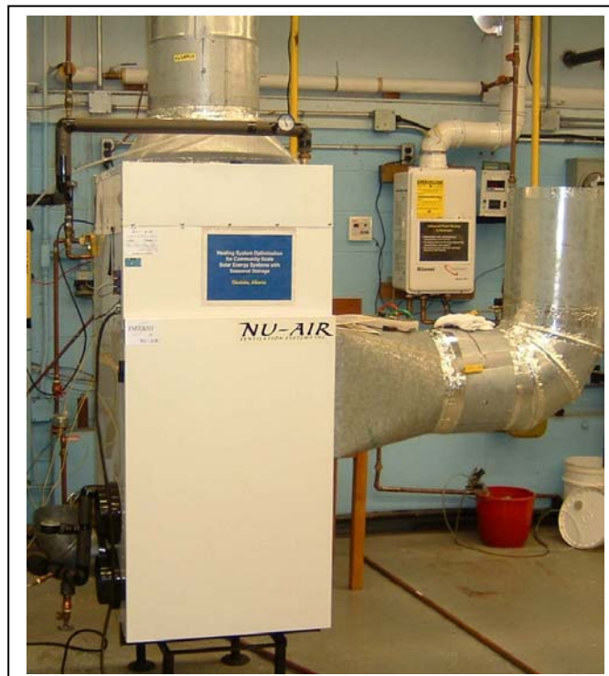
Okotoks- Drake Landing fan coil
