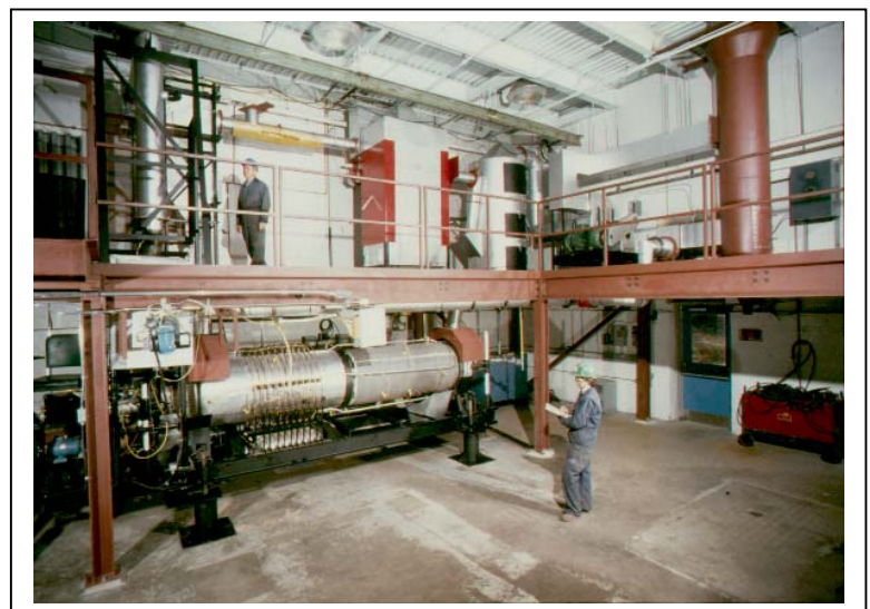
(Fig. 1) 1MW Thermal Rotary Kiln
