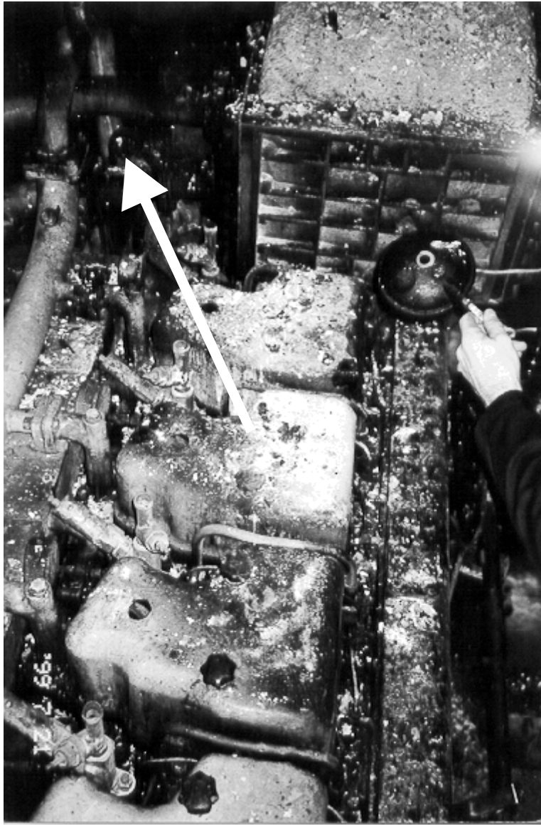
HORIZONTAL CHARRING PATTERN POINTING TOWARDS THE SEAT OF THE FIRE AT THE EXPOSED EXHAUST PIPING
