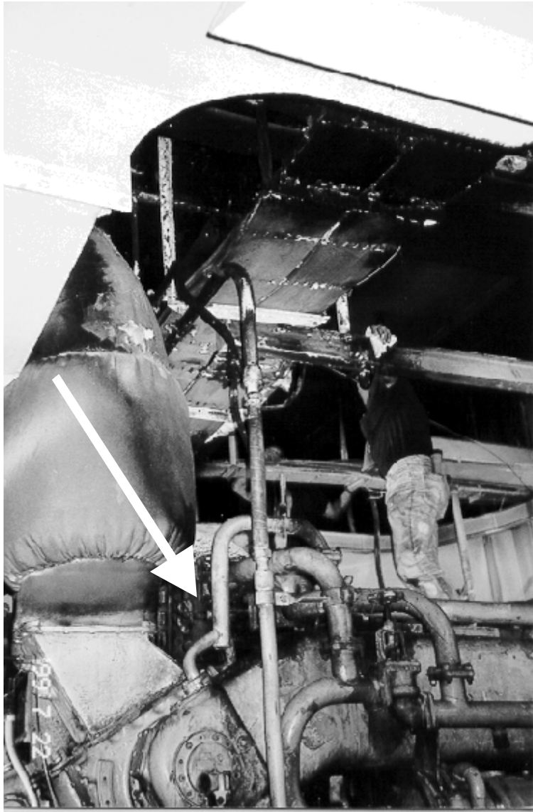
VERTICAL SOOT PATTERN INDICATING THE SEAT OF FIRE NEAR EXHAUST MANIFOLD AT INLET TO TURBO-CHARGER
