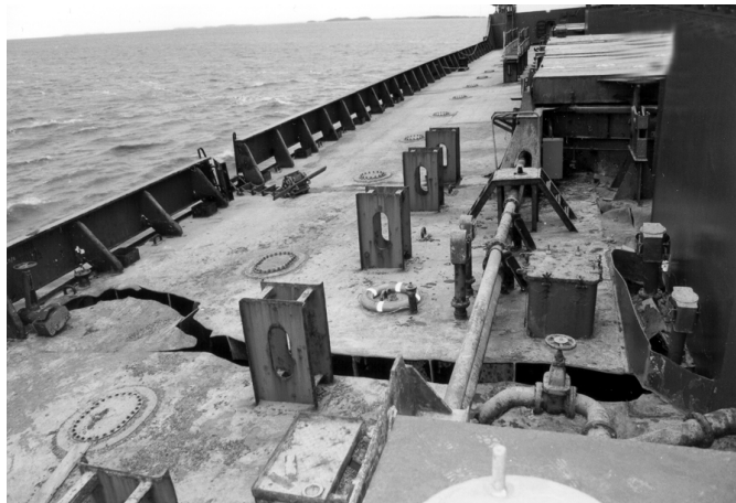
Photo 5. Main deck fracture
