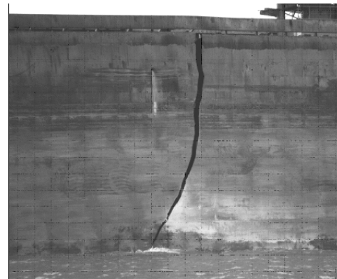
Photo 3. Port side fracture
