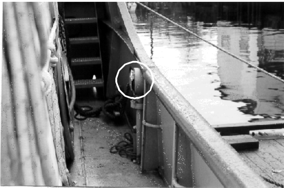
Starboard fuel tank vent (circled) that became submerged during the occurrence and failed to prevent seawater from down flooding into the tank itself.
