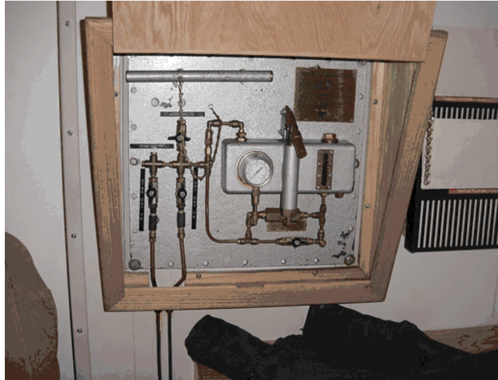
Photo 5. Fuel oil shut-off station
