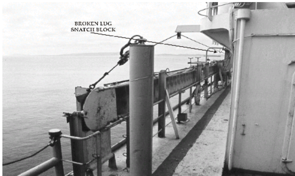
Figure 2. Location of broken pad eye and snatch block.
