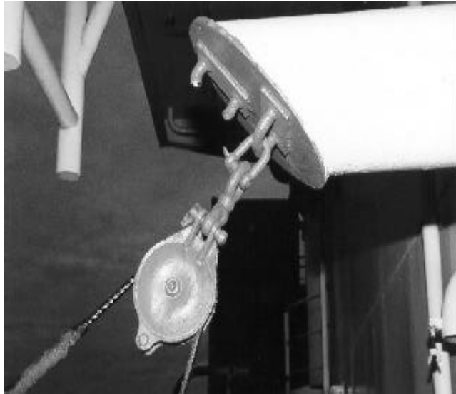
Figure 4. View of broken pad eye.
