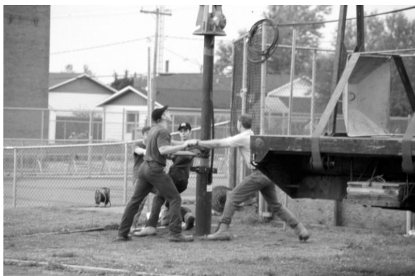
Installation of a high capacity water pump in the production well for aquifer pumping test, north of Montreal.
