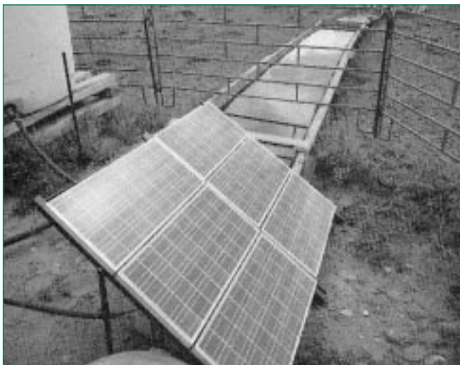
Solar powered water pumping system
