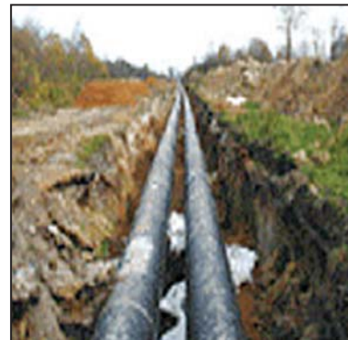
Figure 3: Water Pipes in District Heating System.
