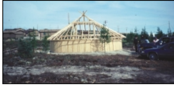
Traditional dwelling under construction in the cultural village beside the new community.
